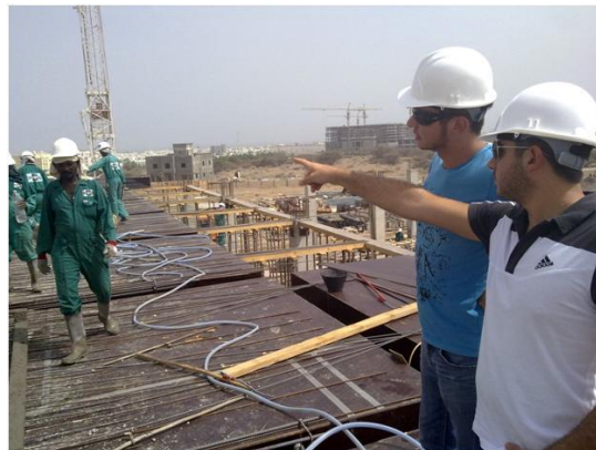
Carl Abi Saab (Electrical Engineer on the right) and Hanna Abi Saab (Civil Engineer next to him) at Bawshar site near the capital Muscat. Concreting of roof and installation of electrical conduits.
