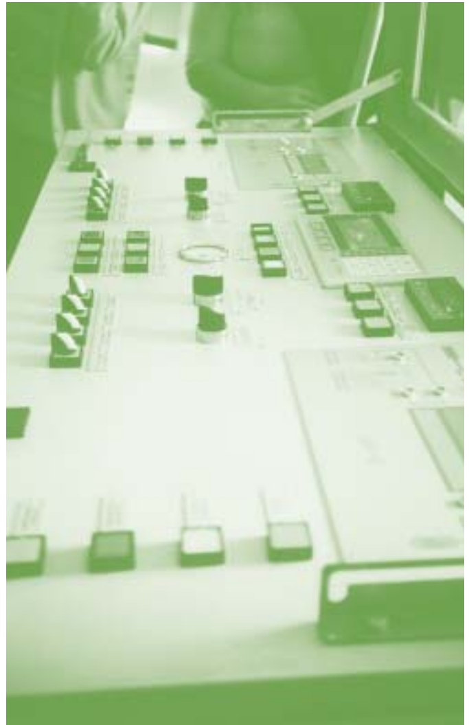
From here the process of purifying the water is controlled.
